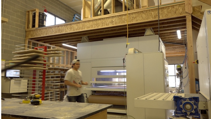
Superfici Mini Plus spray machine performing well in a very tight spot for Advanced Millwork Components & Installations in Lindon, Utah, USA
